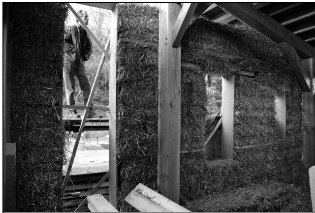
Figure 1. Structural timber framing with non-load-bearing straw bale walls sitting on cantilevered floor joists to provide a continuous insulating external envelope
